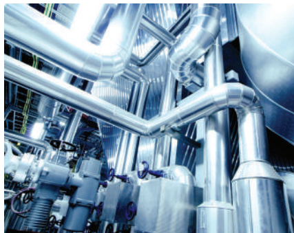
Typical high-corrosive environment — central utility plants.
